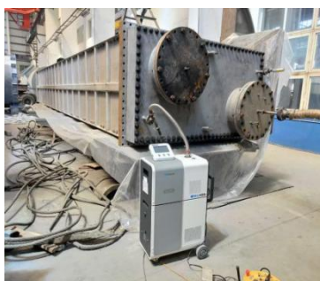
Heat exchanger inspection
